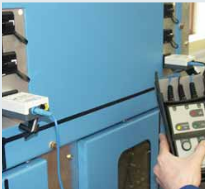
Use of DEHNcap/PC-LRM phase comparator with two HR-LRM test adapters for an HR switchgear installation.
