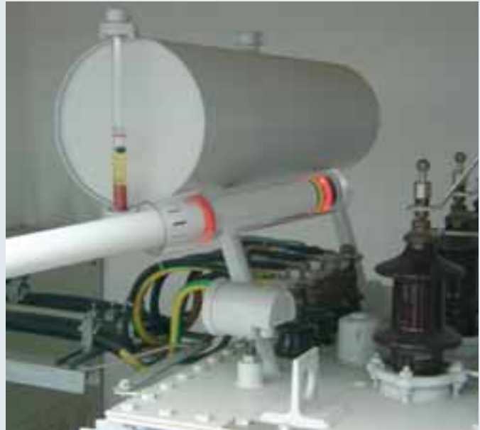
HSA 205 non-contact voltage detector with insulating cap used in a switchgear installation.
