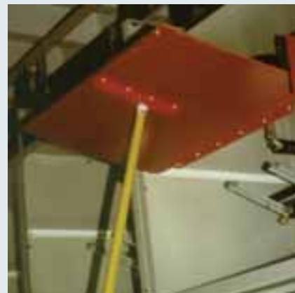
Inserting an insulating protective shutter, type A3, by operating rod
