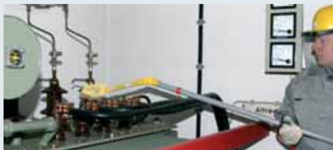
Dry and damp cleaning of a transformer under live conditions using the TFRS MS combined cleaning kit.
