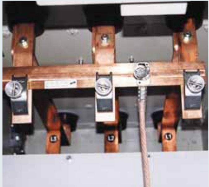
Short-circuiting bar with earthing cable in a switchgear installation.
